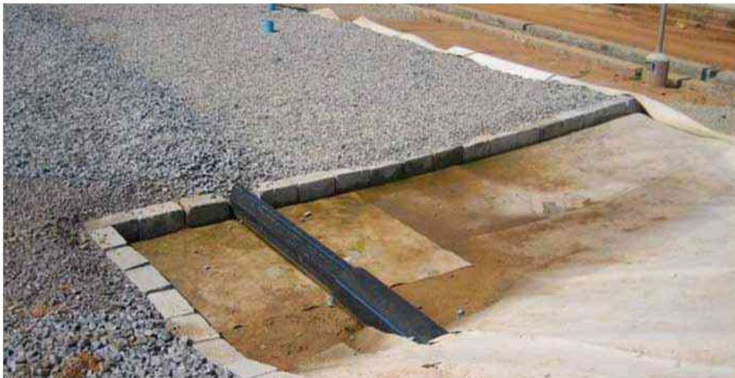
Figure 4.15: Test Field with all Sealing Components 19
