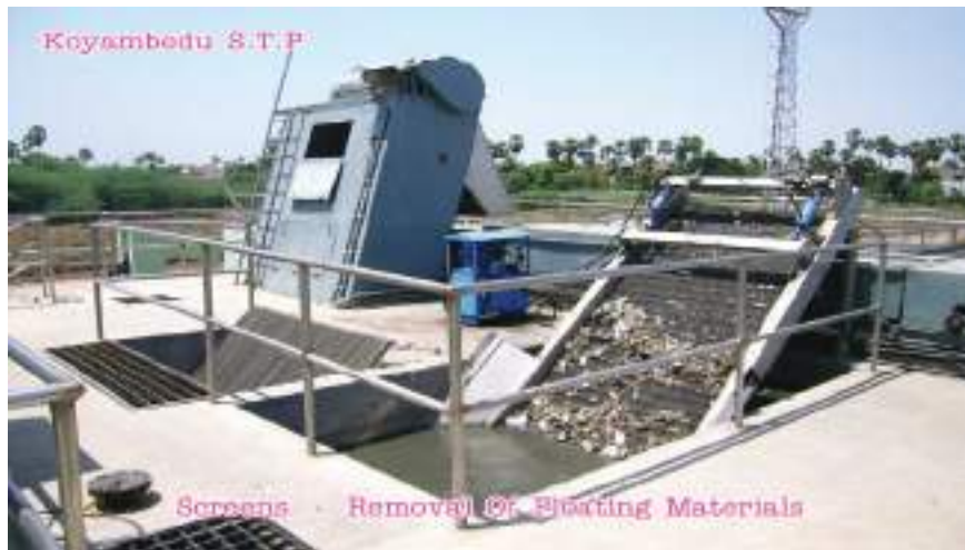
Figure 5.21 Mechanical screen with screen housing and ventilation at Koyambedu STP in Chennai. Manual screen and bypass channel screen in between the mechanical and manual screens is also seen
