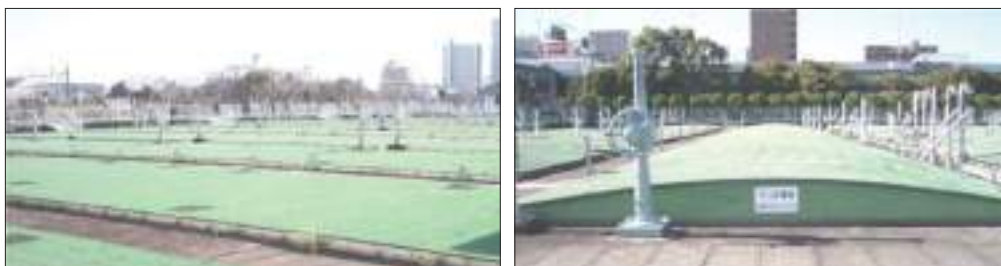
(A) Figure A5.1-1 Covers over sewage structure — Flat type and Dome type (Yokohama City)
