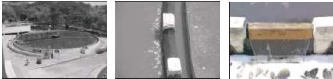
Figure 5.35 Masonry Bevelled Weirs of Primary Clarifiers (left & centre) and Secondary Clarifier (right) with additional entrainment aeration of the treated sewage by the freefall over the weir.
