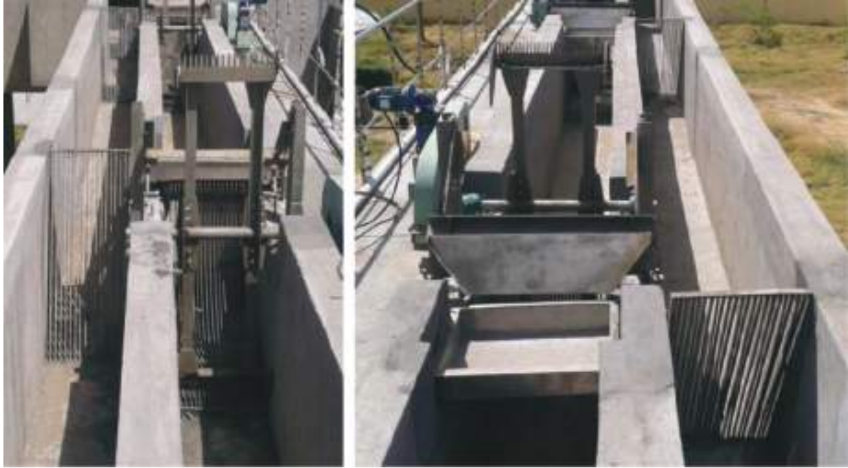
Figure 5.24 UNIDO type circular wedge wire screen seen from upstream at left and from downstream at right in Ramanathapuram STP of Tamilnadu
