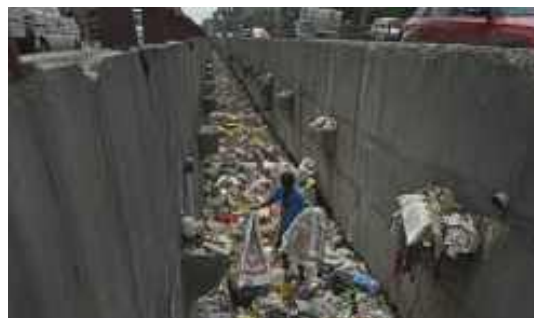
Figure 1.5: Plastic in Storm Water Drain
